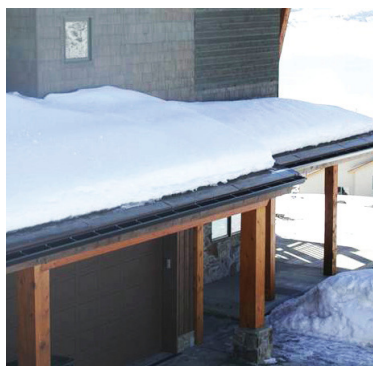
Concealed Roof De-icing
